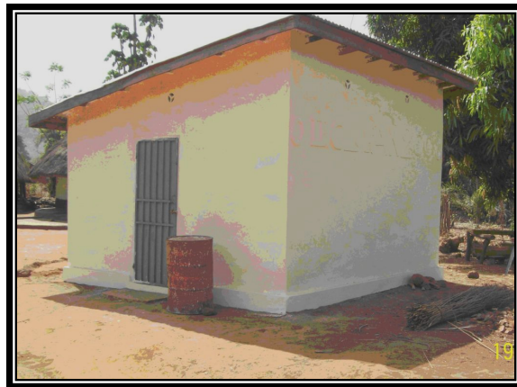
Impact: Reduced Storage Losses. Storage Silo. Source: OICI/G, 2nd Quarterly Report FY09
